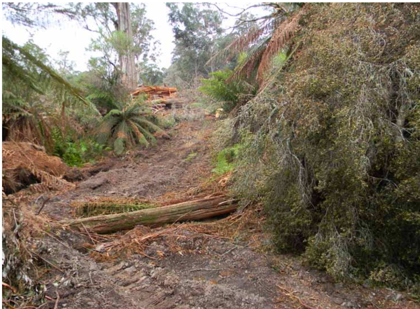
Photo: Bulldozer track that has entered the rainforest gully to push over the mature Black olive berry with a 13.5m X 7.5 canopy width.
