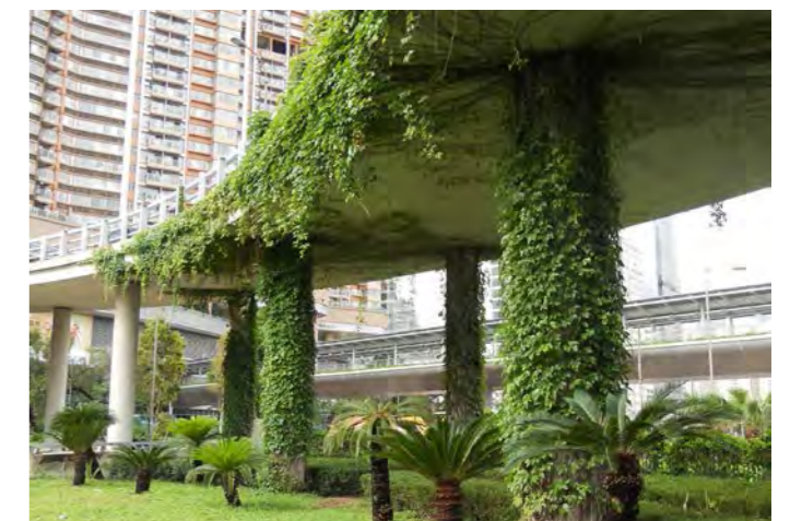
Flyover at Junction of Prince Edward Road East and Choi Hung Road
