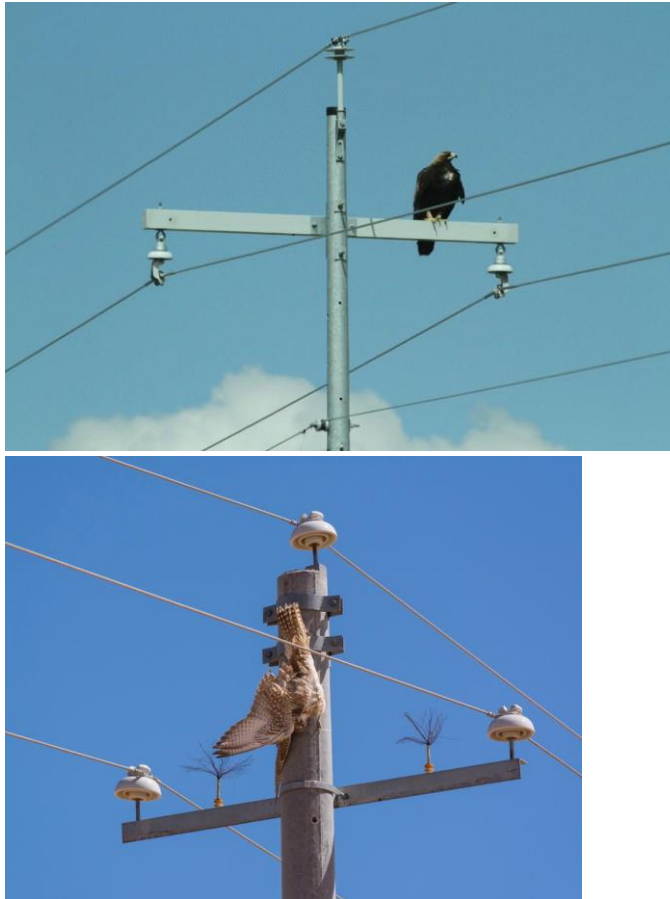
Figure 9-6: Large eagle using transmission line pole as a perch (L) and an electrocuted falcon (R).
