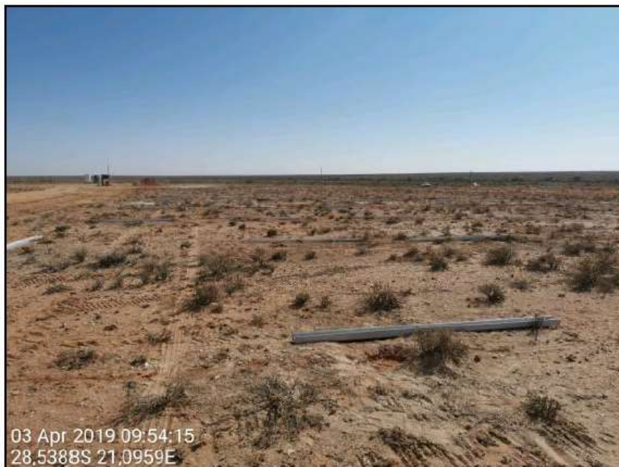
Figure 8: pre-drilled holes are backfilled with a wet sand mixture and steel piles placed in position ready for ramming.
