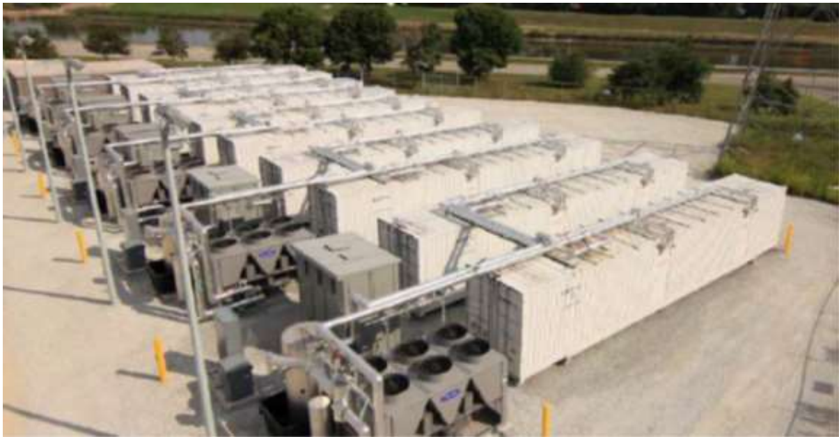
Figure 12: Typical Example of a Battery Energy Storage System.
