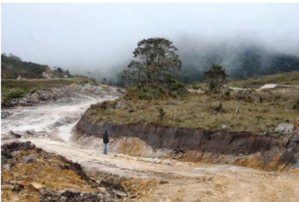
FIGURE 6. A road built in 1998 extends into the subalpine north of Mount Trikora at 3200 m. Built without consultation about conservation objectives it will drain peatlands and provide a nucleus for hunting and fires. Photo by P. Hiscock.
