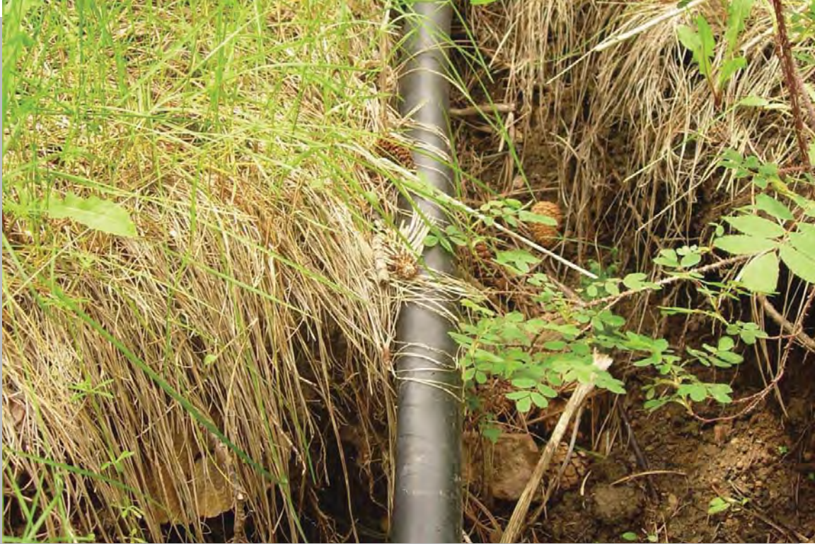
Photo 25 - Water pipe along east boundary of Betasso
