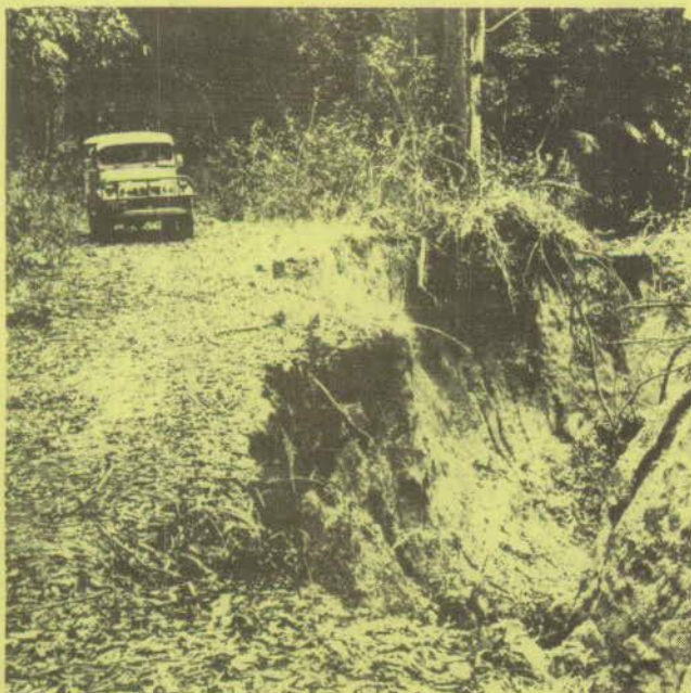
Figure 3 Gully erosion affecting access as a result of poor trail location.
