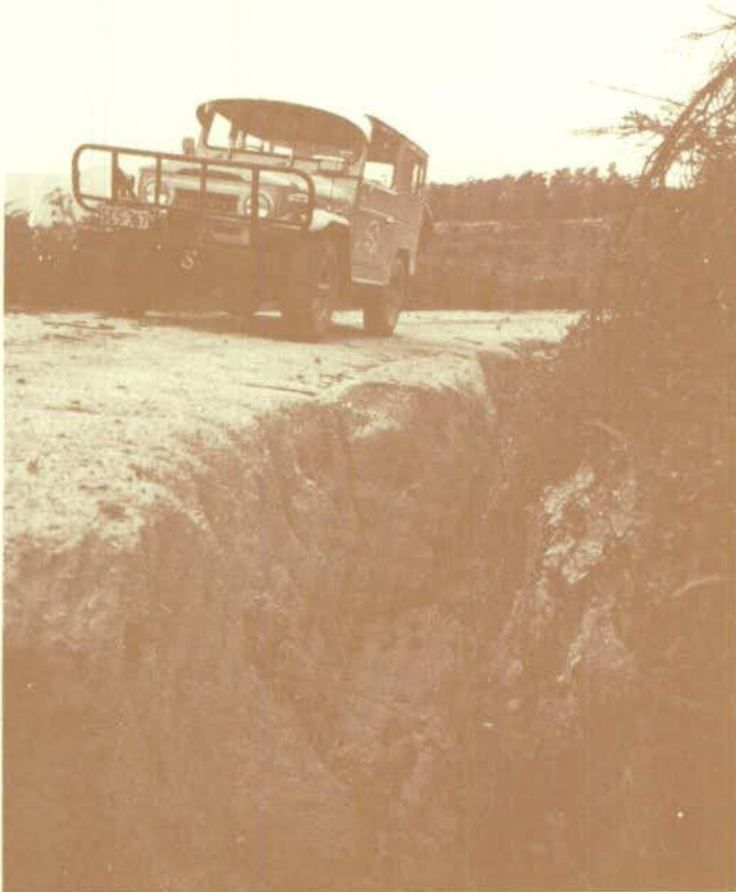
Figure 5 Gullying of table drains is a serious erosion problem and a danger to road users.
