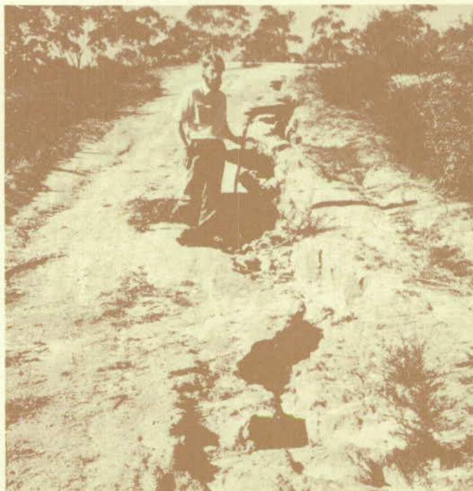
Figure 1 Trafficability is seriously impaired when undrained low standard roads become eroded.
