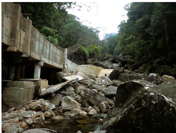
Figure 6. Hydroelectric power plant (note: concrete wall built across the stream and concrete particles dump into the stream).
