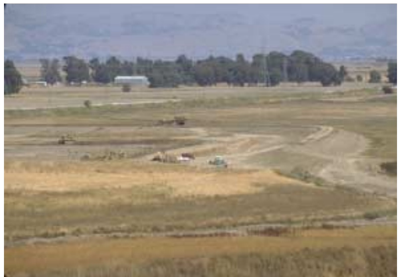
Over 400 acres of tidal wetlands were restored along Tolay Creek in December 1998 (shown here in construction phase).
