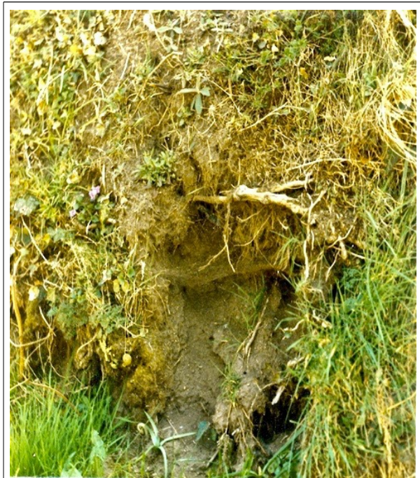
FLAIL DAMAGE : A poor photograph, taken early in the year (March 1982) on north-facing hedge of the survey lane. Shows holes near foot of hedge where large stones have been dislodged by flail, dry earth now sliding out from dust-dry core.
