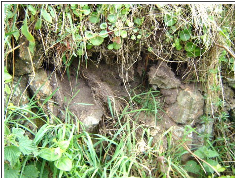
FLAIL DAMAGE. Centre stone knocked out by flail at first flailing, then one either side the following year, then two fell from centre of row above, followed by one more knocked from centre row and four more from row above as they slumped forward. Next stone to go, second from right, centre row. Fine earth from dehydrated core of hedge sliding out over stone at left of gap.
