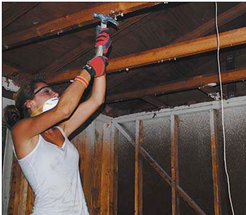
Melanie Digrigoli, 15, of Indian Rocks Beach, pulls nails while working to strip a local home of storm-damaged drywall on Thursday.
