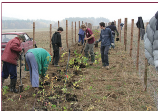
Fig. 2. Planting of a hedge upstream of the Chocholouš pond. (Archive Czech Union for Nature Conservation, Vlašim)
