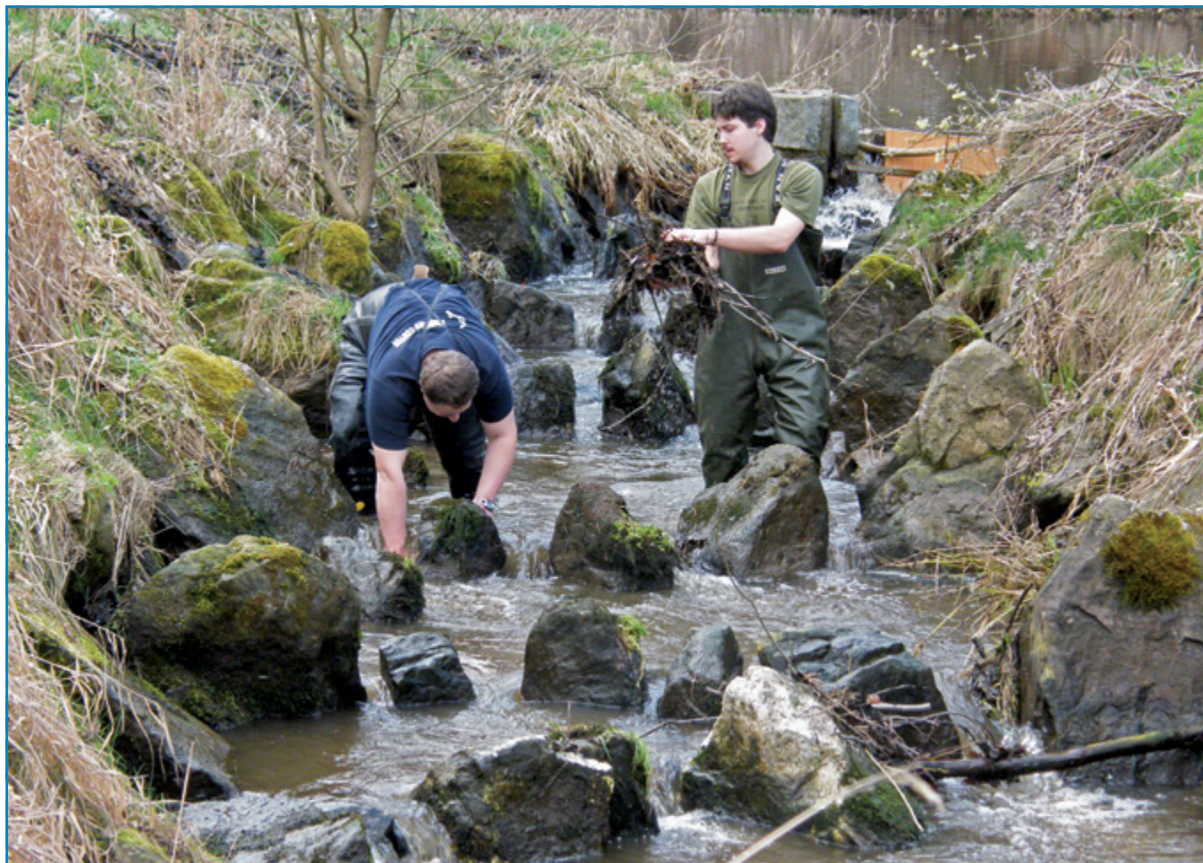
Fig. 4. Removal of sediments and objects from the bypass during reduced stream flow. (P. Dvořák)
